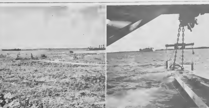
THIS IS the site where the chemical complex at Baredera will be constructed. At right is the business end of the enter-suction dredge "Barlow," which is expected to finish the industrial harbor dredging operation in about three months.
